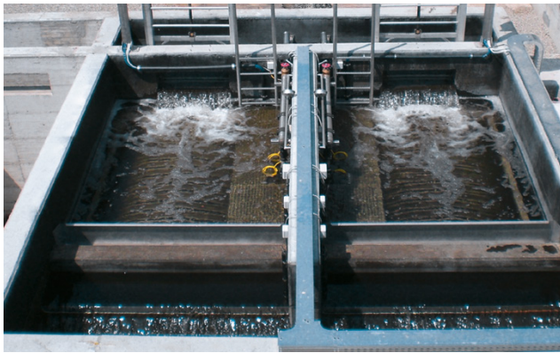
Passavant® PCF® after secondary clarification
