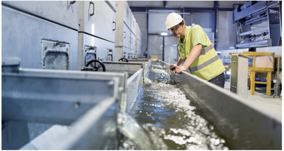
Power Plant Intake in Europe: Geiger® MultiDisc® with Fish Trough and Cover Panels
